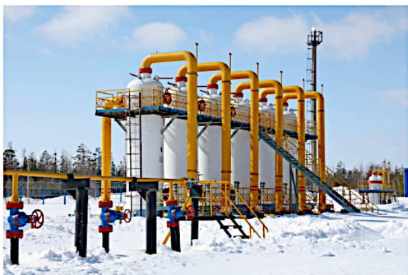
Natural gas storage facility in Russia
