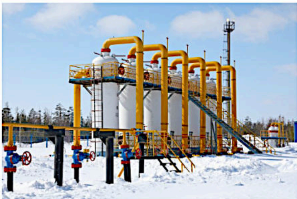
Natural gas storage facility in Russia
